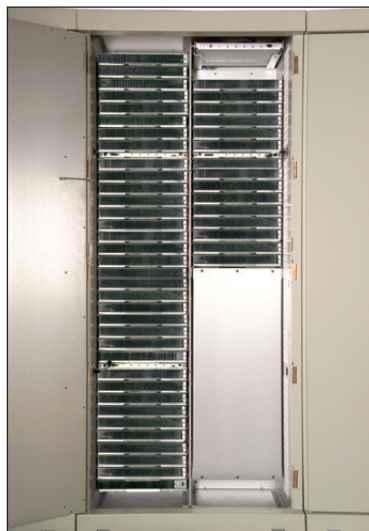
RF modules may be removed while on the air
